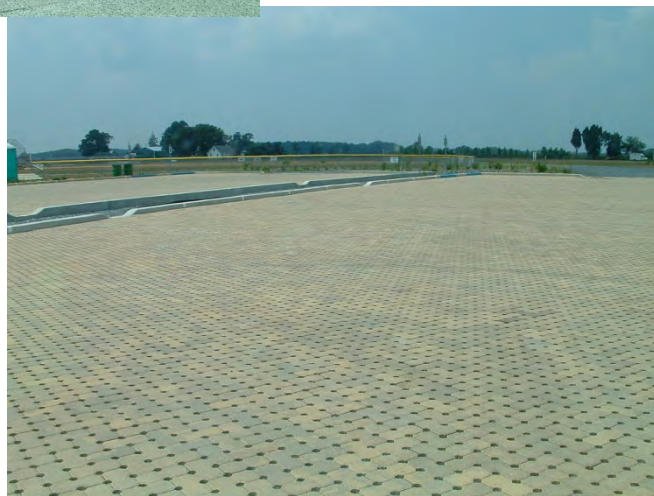
Bloomfield Parking after - Permeable pavers allow runoff to soak into the soil below and prevent heated and fast water from negatively impacting local waters.
